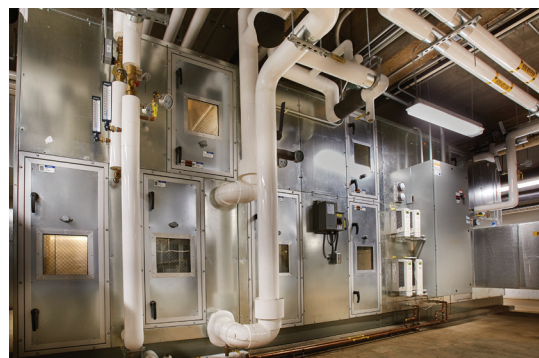
One of four Innovent units installed at the University of Minnesota Aquatic Center
