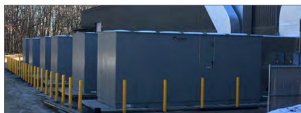
Six grow room air handlers mounted outdoors
