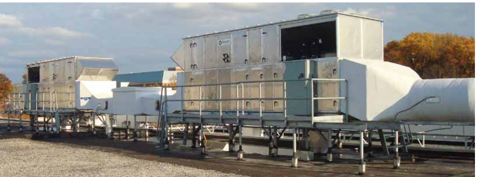
Two Innovent Natatorium Dehumidification Units (NDHU) on the Burdick Hall roof.
