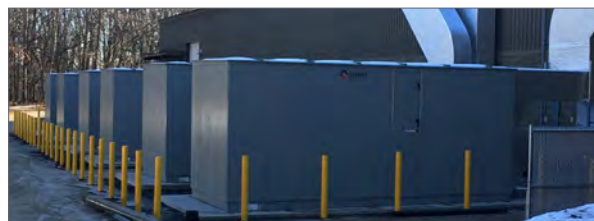
Six grow room air handlers mounted outdoors
